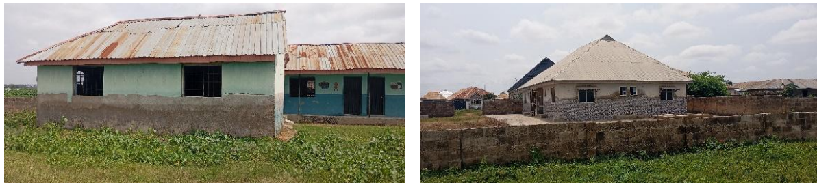
Figure 2. Waterlogged conditions around selected buildings within the Asa River wetland corridor, Ilorin. The photographs document saturated ground and visible indications of previous water exposure on structures located close to the wetland. Source: Author's field photographs, [25 August, 2025]
